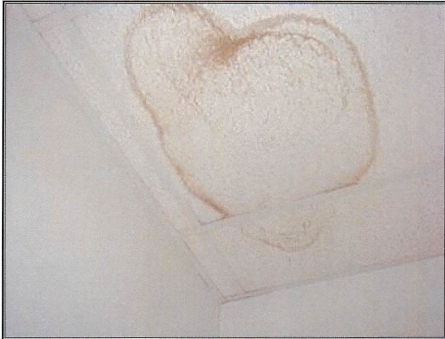
Noted water stain in 2 nd floor restroom
