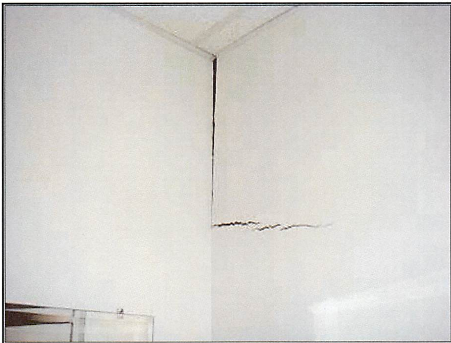
Noted deferred maintenance in subject building
